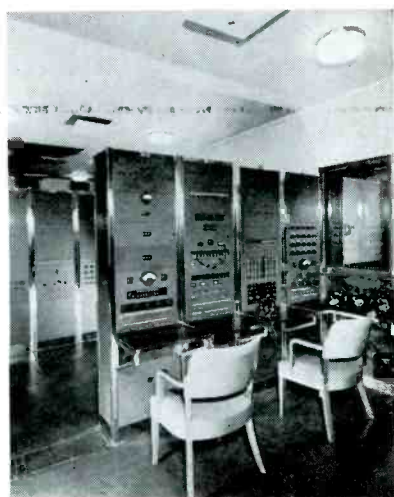
Output switching panel in WWJ Main Control Room.
